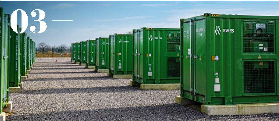
BW ESS: Charging ahead in battery storage
